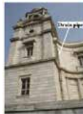
Fig-10: Drain pipe
