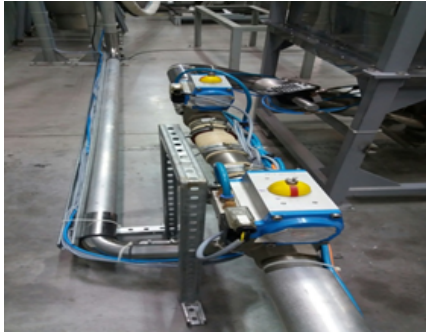
Figure: 3 – Automatic system of silos
