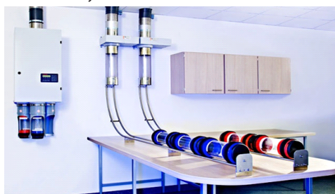
Fig 8: Pneumatic tube transport system
