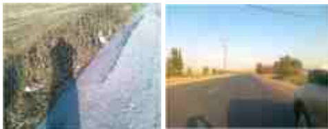
Fig.3 Cracks seen on the roads Fig.4 Cracks seen on the roads
