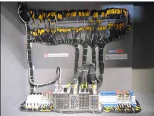
Figure 2. Vehicle Control Unit and expansion modules inside the TCMS simulator
