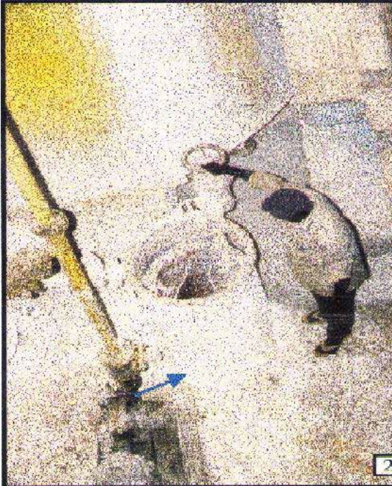
FIG.7 LIME STIRRER UNIT NEAR LIME SLAKER NOTE THE HIGH CONCENTRATION OF LIME DUST AND WORKER WITHOUT PERSONAL PROTECTIVE EQUIPMENT.
