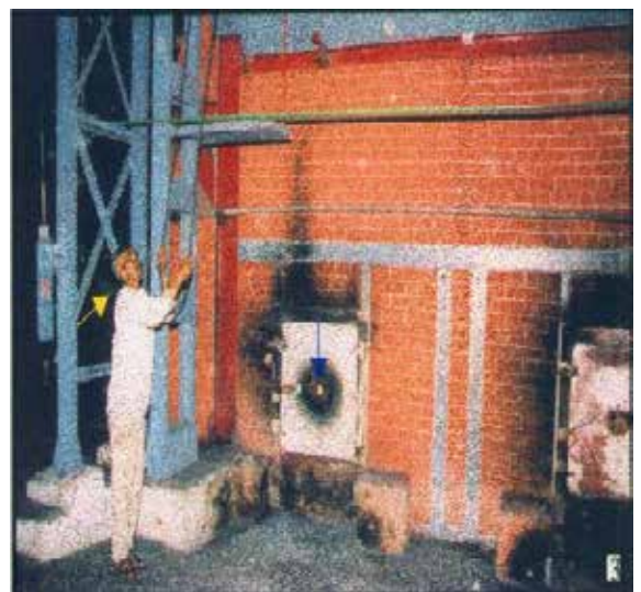
FIG.3. WORKER IN CLOSE VICINITY OF BOILER NOTE THE EXCESSIVE HEAT AT THE WORKPLACE AND WORKERS WITHOUT PROTECTIVE CLOTHING.
