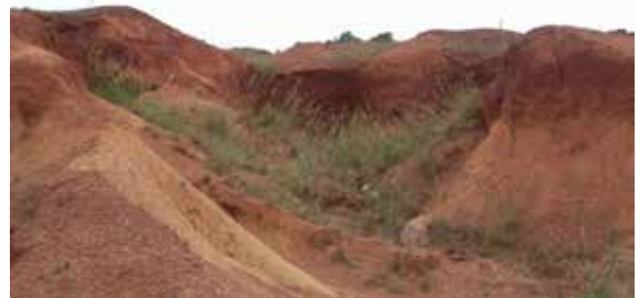
Plate-1: Second level tramped shaped gully with some deposited material on its bed in Rangamati Gully Basin
