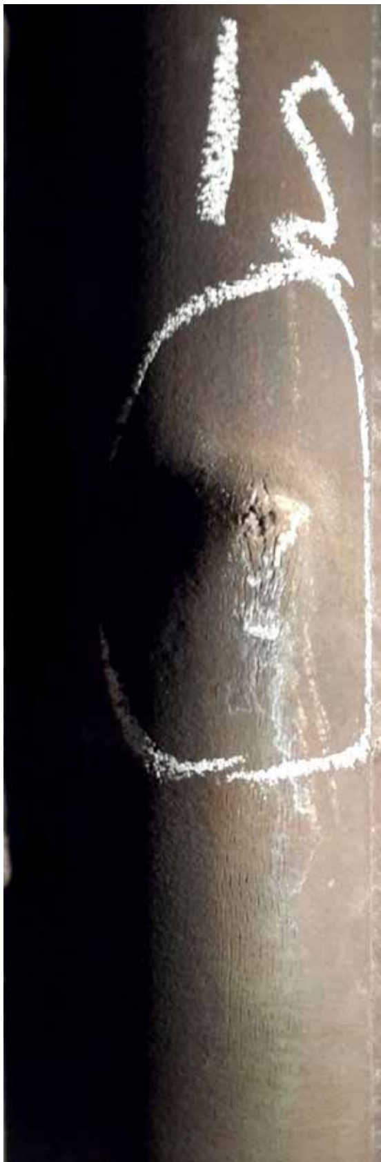
Fig. 3 : Failure of Platen Super Heater Tube
