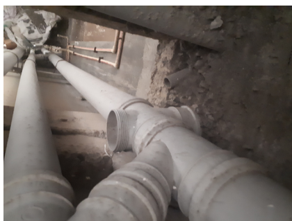
Fig- 4 Actual pipe network in building (Source:-Prateek Group site visit)
