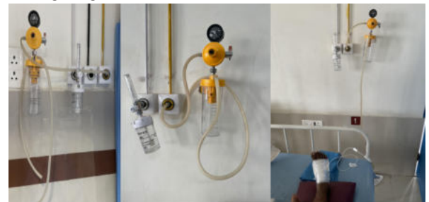
Figure-2,3,4: Hospital central suction device.
