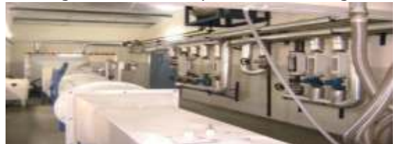
Fig.9 Rotameter & heater used for lubrication temp and flow management.
