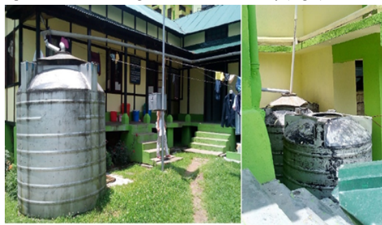
Fig 9: Rain water harvesting tanks in the College Hostel
