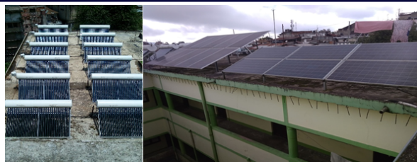
Fig: 3 Figure of solar powered water heaters and solar powered lighting systems
