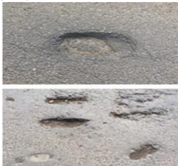
Fig.1 Example of pothole
