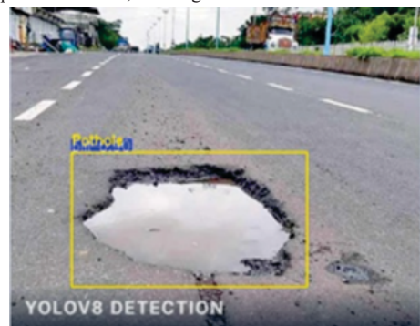
Figure 1: Pothole Detection using YOLO Model
