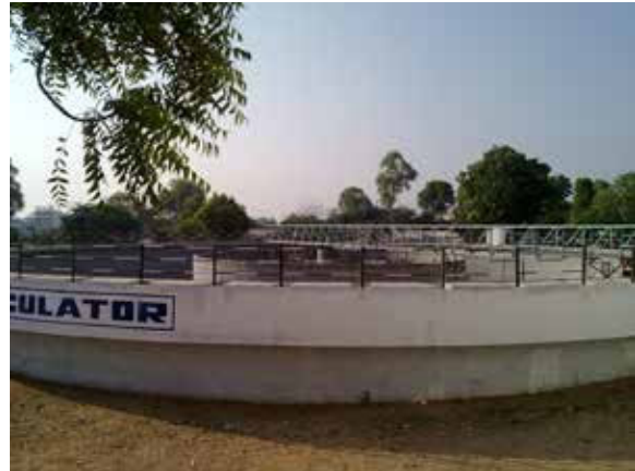
Figure-3 Water Treatment Plant at Siddhi Sarovar
