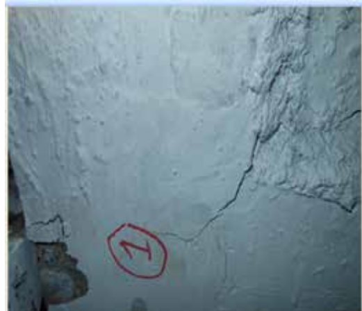
b) Final crack appear in mortar back side view
