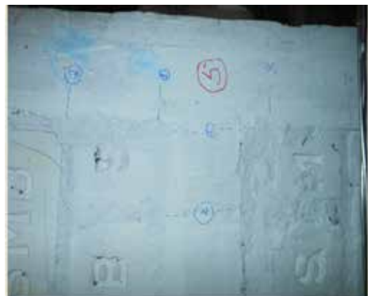
d) Final crack appear in mortar front view
