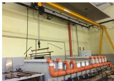
Figure 2 Production line of surface treatment
