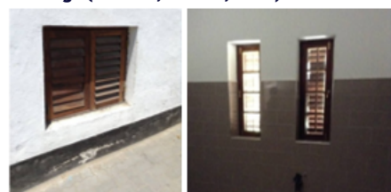
Figure 10 and 11; Openings that face a major high way and cause Noise inside the building.
