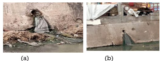
Figure 3: Domestic wastewater discharges to Canal IV
